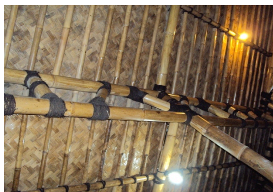
Detail under the roof showing the manner in which the bamboo pole elements of the roof framework are connected with one another
