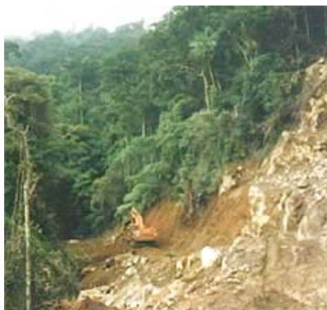
PNOC cleared the forest in Bgy. Mailoum for road building so they can prepare for their entry in the strict protection zone.
